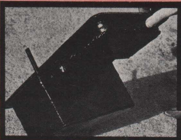
4: The cut and welded sump pan with the new section fitted in which tucks down between the frame tubes.
