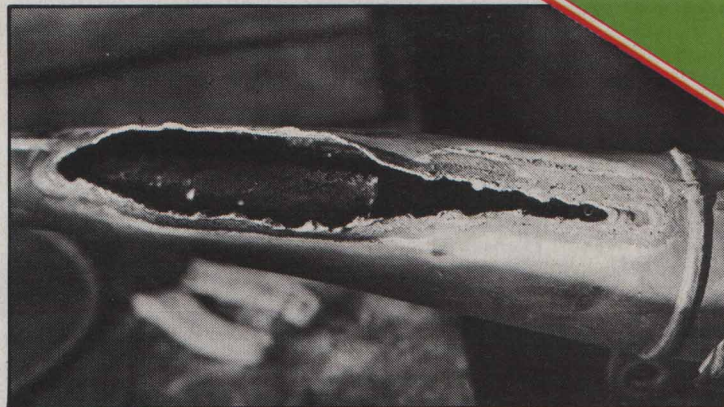
Pipe cut open to show extended primary pipe which has to be cut out.
